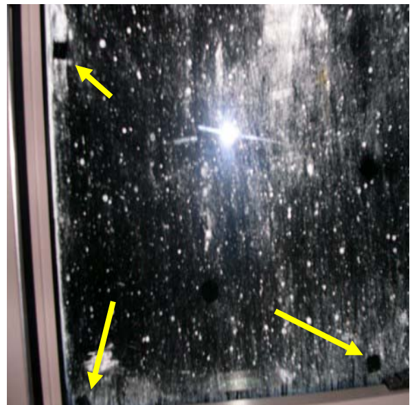
Photo Above shows an installed window with heavy condensation on Glass. Different patterns are visible within the condensation including the outline of separator pad marks on glass. As above there are no visible marks present on this glass in the absence of condensation.
