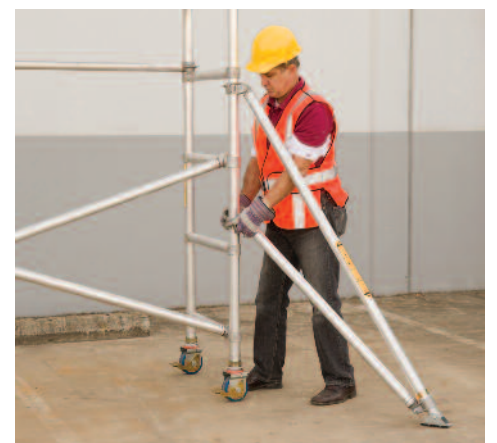
3. Before moving platform higher than 7ft. (2.1m), tie the scaffold into the building or install outrigger on each corner. Make sure each outrigger is wedged against solid pavement and that all couplers are securely fastened.
