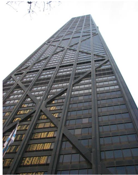
John Hancock Center has both bronze anodized aluminum and black anodized panels. Years of oxidation appears as white haze and streaks.
